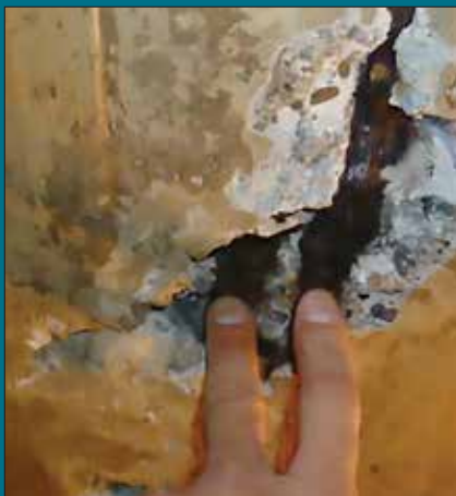
Photos show delamination and loss of integrity of walls and water bearing structures and roof patches.
